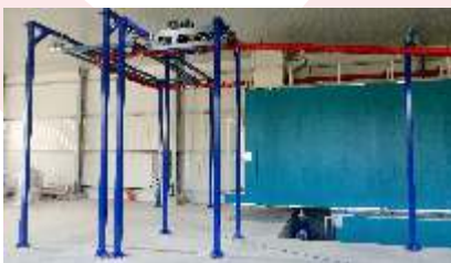
Conveyorised Powder Coating Plant
